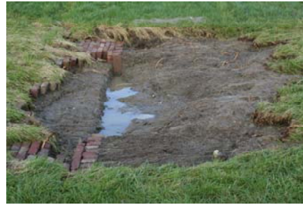
Figure 10. Damage at transition from slope to horizontal; 50 l/s per m
