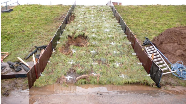
Figure 6. Failure of section 4.
