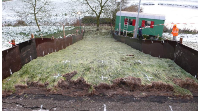
Figure 3. Final result test section 1, looking down the slope; minor damage at transition asphalt road to grass covered slope 1:4.
