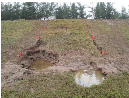
Figure 7. Failure of a Bermuda grass slope, section TL_01.
