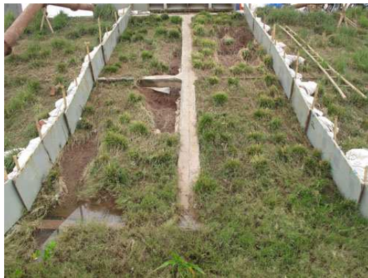
Figure 6. Various damages on a mixed grass slope, section TT_03.
