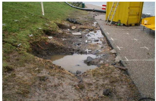
Figure 10. Final damage after the pilot run-up test.
