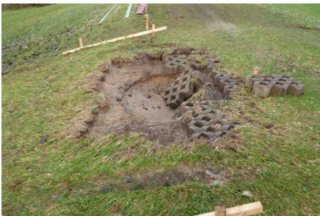
Figure 8. Failed road crossing by under-mining due to simulated wave impacts.
