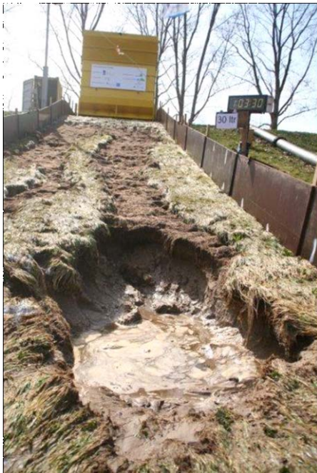
Figure 15. Failure of a sand dike.
