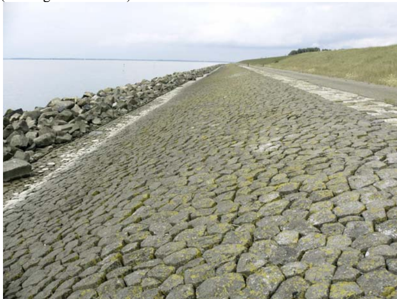
Figure 1. A dike with a rough rock berm around swl, smooth upper slopes, including a smooth berm
