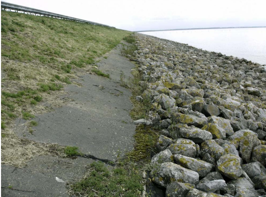
Figure 13. Prototype profile 2. Berm at swl and one layer of rock on smooth slope
