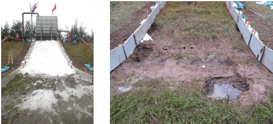
Figure 5: Rough guidance of overtopping flow (left) and damages (right) at dike toe, TL_01.
