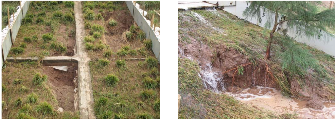
Figure 9: Left: damage around concrete frames. Right: damage extension to the Casuarina tree.
