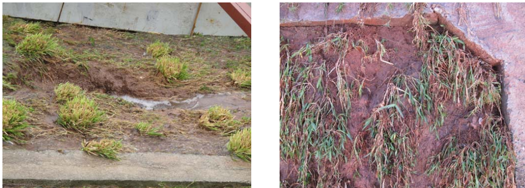
Figure 8: Left: damages amongst Vetiver clumps. Right: poor cover of Bermuda grass and settlement of soil around concrete beams,
