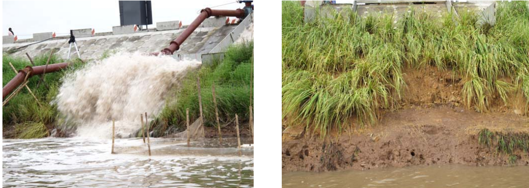
Figure 6: Overtopping flow flying from the berm attacks the dike toe.
