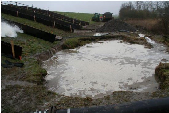
Figure 6. Scour hole at the toe of the dike; the sub soil consists of gravel (Kattendijke)
