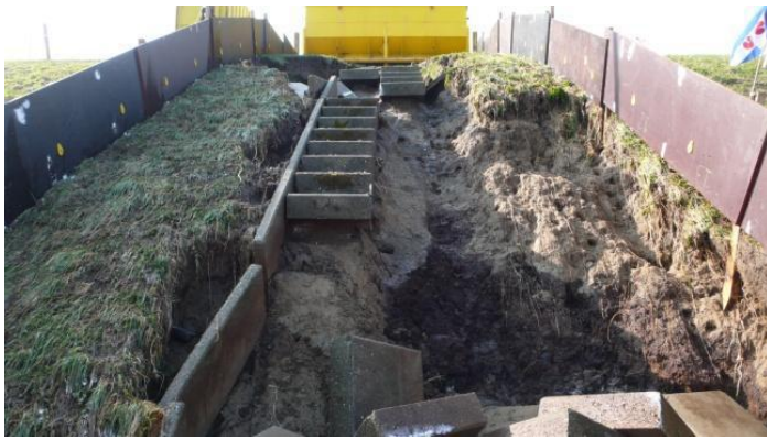
Figure 8. Erosion close to stairs (Tholen)
